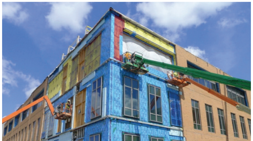
FIGURE 2 Design reviews, mock up coordination and early performance testing by the BECxA can identify problems and provide solutions, minimize design and installation deficiencies, and mitigate the potential for enclosure-related failures.
